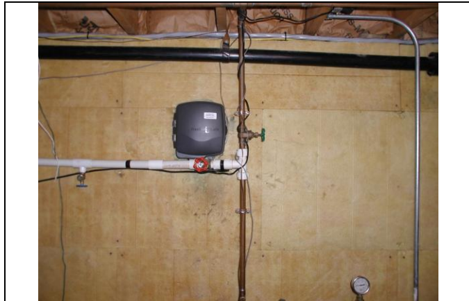
Figure 13 A lawn sprinkler addition made of PVC pipe interrupted the water pipe ground path with a plastic tee that needed to be jumped around.
