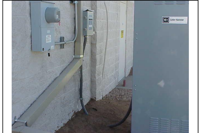
Figure 16 Long wiring loop between TVSS and electrical cubicles causes an excessively high let through voltage.
