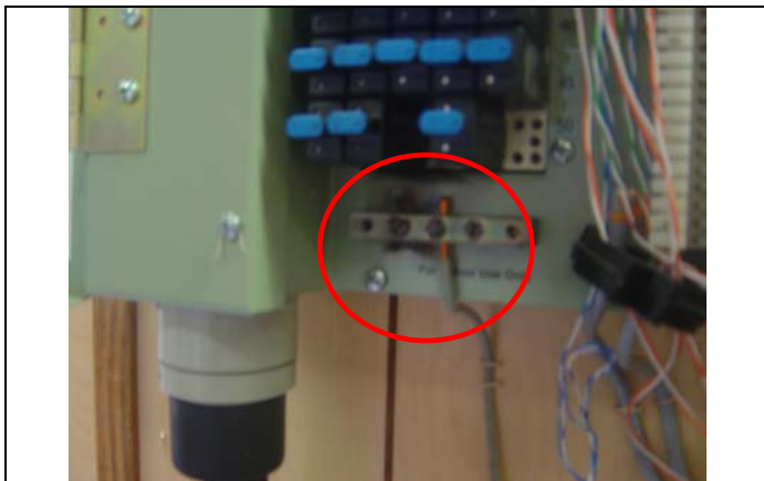
Figure 21 , a poorly grounded protector mounting. Note the Flashover burn evident just behind the grounding bar to the left of the wire.
