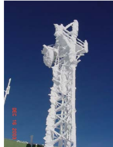
Figure 4 Heavy ice encrustation on a tower can fall away in large chunks posing a threat to unprotected equipment below.
