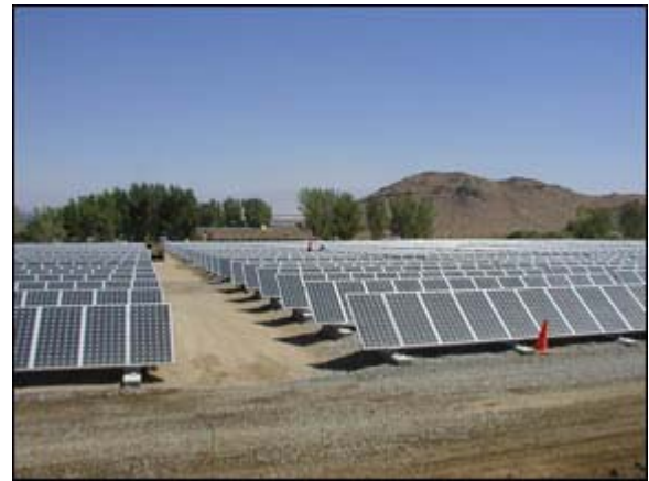
Figure 10 A large scale photovoltaic system
