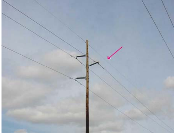
Figure 12 A grounded catenary wire (Arrow) protects a power transmission line from lightning.
