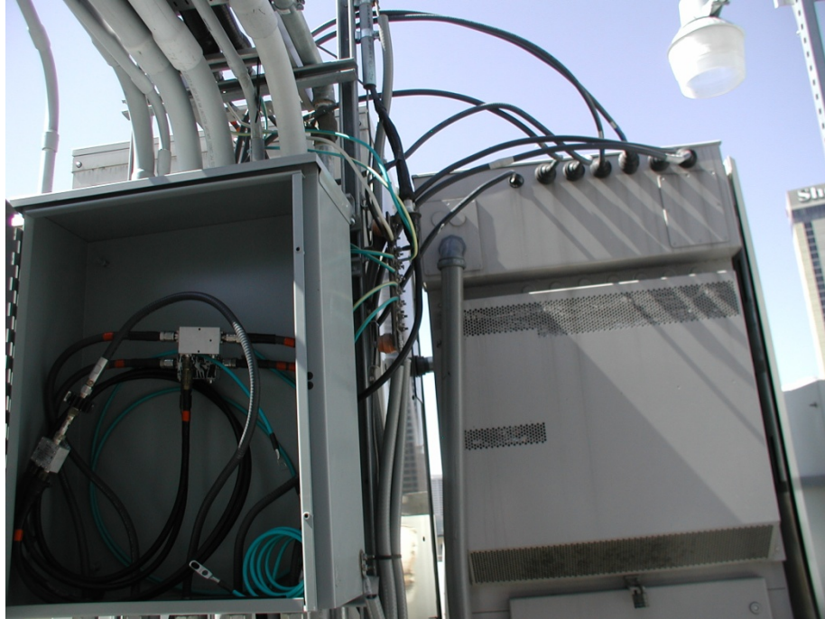
Figure 2 Rooftop cell and microwave sites have larger quantities of easily stolen copper wiring than do ground level sites, and increasingly these rooftops are being targeted by metals bandits.
