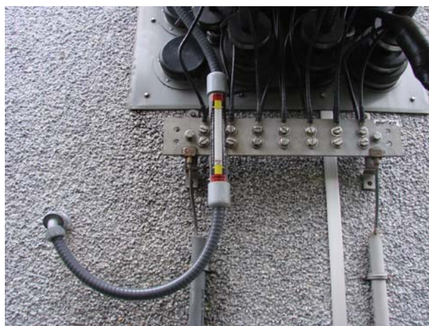
Figure 17, one method of alarming a ground bar.
