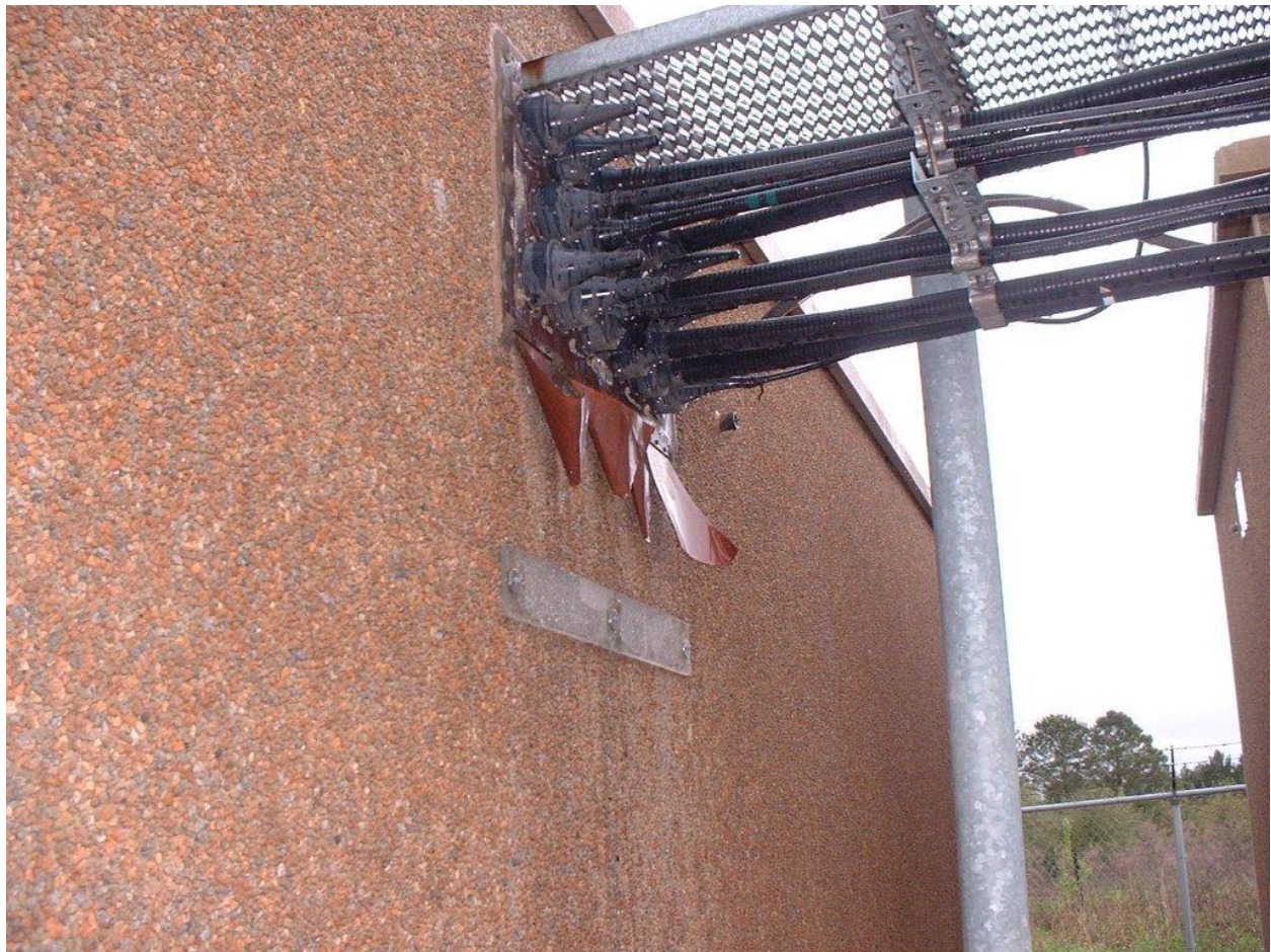
Figure 1 depicts four cut copper ribbons that once connected the hatch plate and the ground bar just inside the hatch plate to the buried Ground ring.
