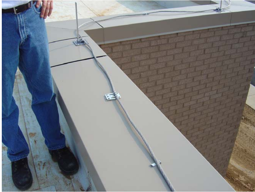
Figure 7 if aluminum wiring is adequate to provide lightning protection for a building, why then shouldn't aluminum conductors also suffice to bond and ground the systems and subsystems for a rooftop cell or microwave site? (Note: the system shown here is still being constructed; hence some of the connector bases aren't tightened yet, nor are the anchor plates cemented down with silicon sealer.)
