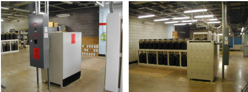
Figures 1 and 2. Cabinetized VRLA batteries share a spacious power room in this UPS application.
