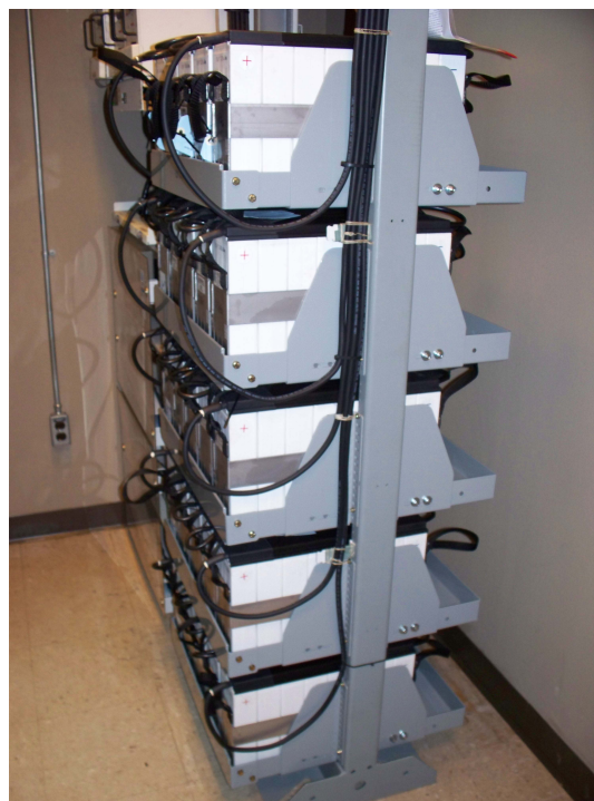
Figure 1 a NiCad battery used in a shelter application permits operation without refrigeration based HVAC, therefore cooling cost is reduced and ventilation is increased
