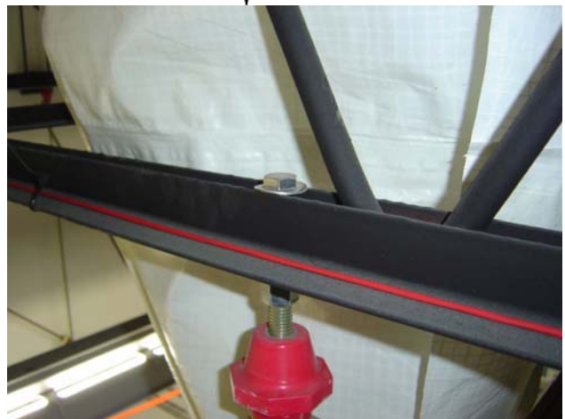
Figure 8 when supporting from overhead truss joists fender washers are inadequate and thick rugged washers are needed to prevent pull through failures. Note the bowing evident in the washer pictured and in the illustration.
