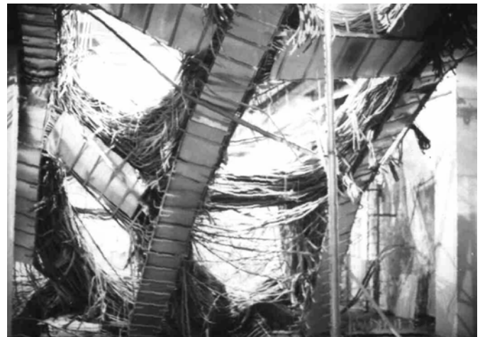
Figure 19, a serious cable rack collapse can occur if too many of the supporting frames are removed.
