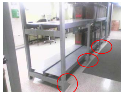
Figure 20 a type of battery stand that experienced failures during a US earthquake. The failure points are identified by circles.
