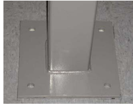
Figure 15 Stanchion lacks floor connection
